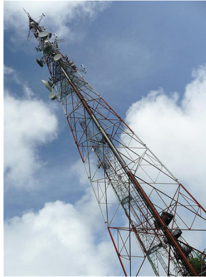
Figure 12.4.1 - An example of a telecommunication facility tower.
