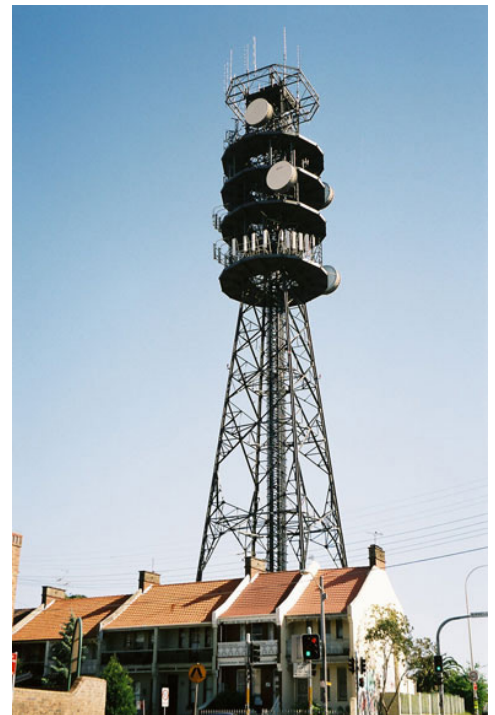
Figure 12.3.1 - An example of the negative visual impact of a tower on neighbouring houses.
